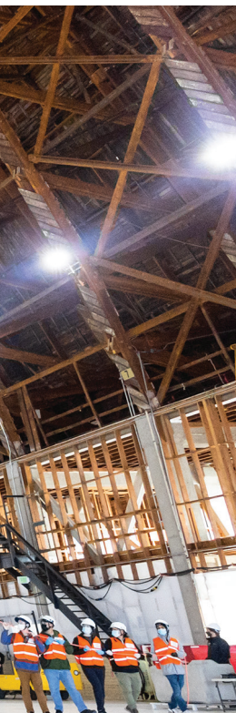
LTA Research staff maneuver Pathfinder 1 while the airship is under construction at the company's Moffett Field facility, near San Francisco.
