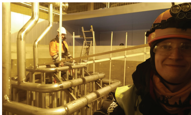
FIGURE 4 Tommi Eronen (foreground) and Ylönen inspecting the ductwork of a Polar Night Energy heat storage vessel.
