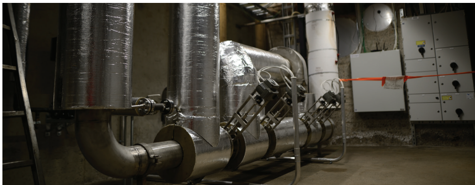
FIGURE 7 Part of the heat transfer system installed by Polar Night Energy in Tampere, Finland. The vertical pipes at left are part of the heat exchanger, while the resistive heater elements are wrapped in white insulation at right. Between these components is the air-circulating radial blower.
