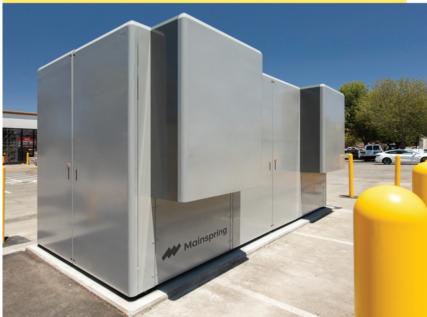
Mainspring Energy's first commercial product contains two linear generator cores. This unit, installed outside a store in Northern California, can produce up to 230 kilowatts of power.
